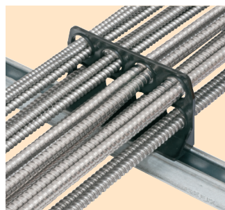
CA8L on unistrut, power cables
